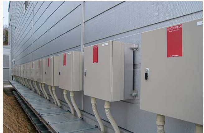
PV Inverter at Fujiyama Works
